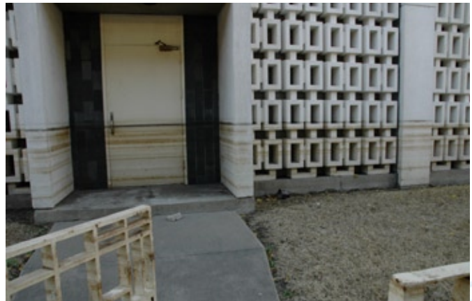
Stains on the walls of the building show the water level on the Delgado Community College campus.
